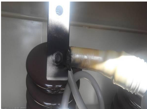
35KV开关柜电缆头短路烧损
