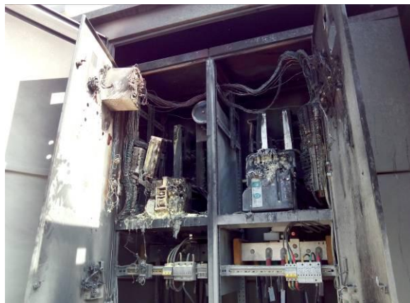
箱变低压柜烧损
