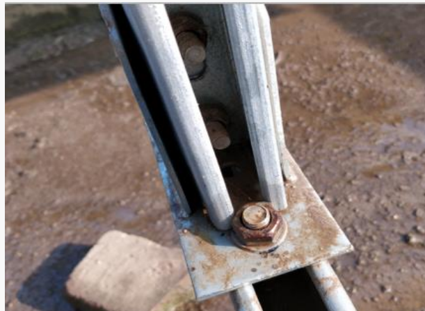
螺栓锈蚀且过短
